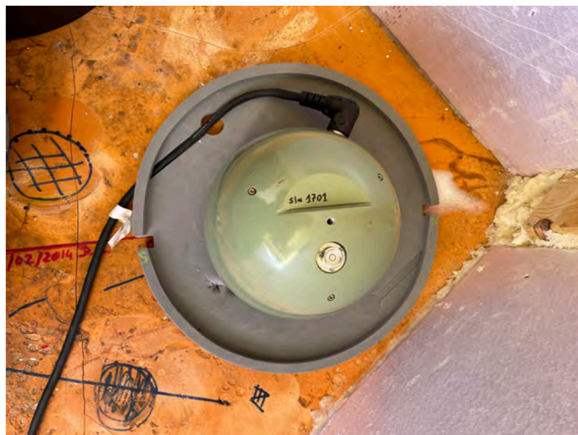
Seismograph installed in PEA’s GEOS scientific shelter.
